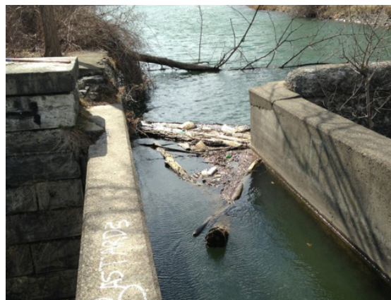
Limestone aqueduct over Limestone Creek showing debris blocking flow
