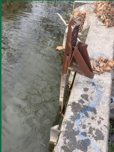
Control Structure (closed)
