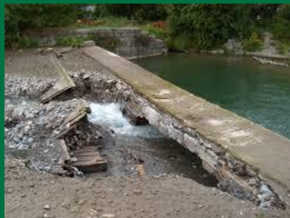
Weir undercut and thus removed
