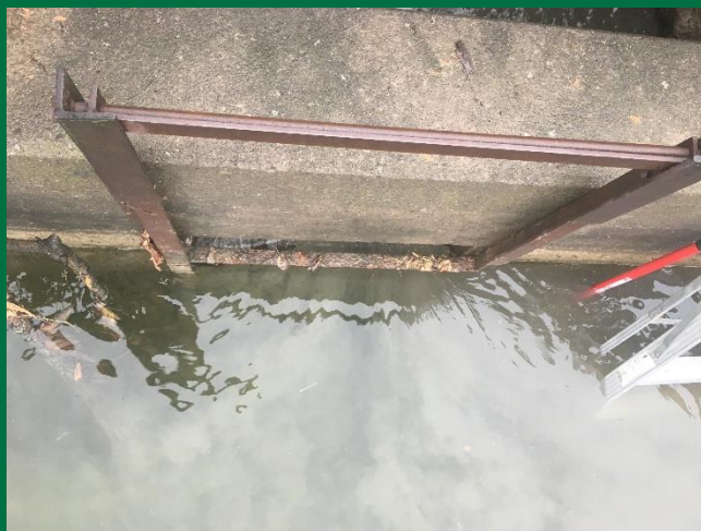
Outfall gate partially closed with flashboards
