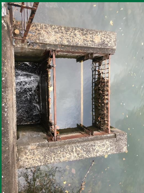
2 sets of flashboards
