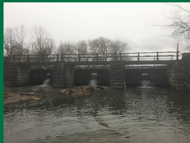
Considerable amount of water lost
